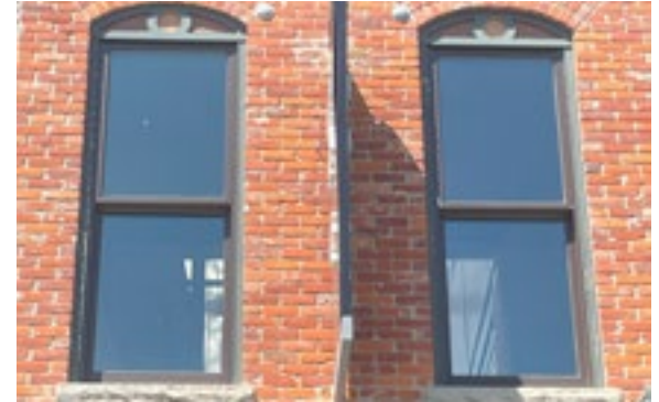
If replacement of historic windows is necessary, replacement windows should maintain the historic window's features such as glazing pattern, profile, and dimensions. Photo by KDG, 2023.
