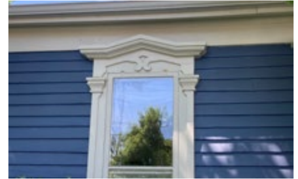
Storm windows provide additional thermal efficiency and protect the historic windows from the weather. Photo by KDG, 2023.
