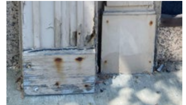
Adequate maintenance of historic buildings involves periodic inspections to ensure historic features are well maintained. In the image above, the peeling paint and rust spots on the wood trim indicate water infiltration that needs to be addressed. Photo by KDG, 2023.
