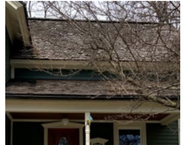
Wood shingle roofing is fairly common in Northville's Historic District. These roofing materials should be retained and preserved. Photo by KDG, 2023.
