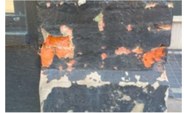
Painting unpainted masonry is not appropriate as moisture can become trapped in the masonry, leading to spalling as pictured above. Photo by KDG, 2023.
