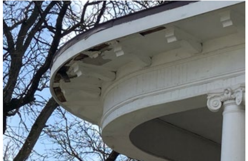
Repairing and maintaining character defining features on this porch, like these brackets, columns, and other wood features is an appropriate practice. Photo by KDG, 2023.
