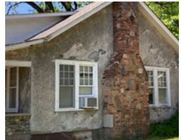
Large portions of missing stucco may require re-stuccoing the whole wall rather than discrete patching. Photo by KDG, 2023.
