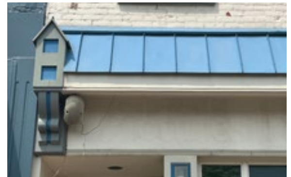
Unless metal roofing was used historically on the building, the incorporation of metal roofing materials onto historic commercial buildings is not appropriate. Photo by KDG, 2023.
