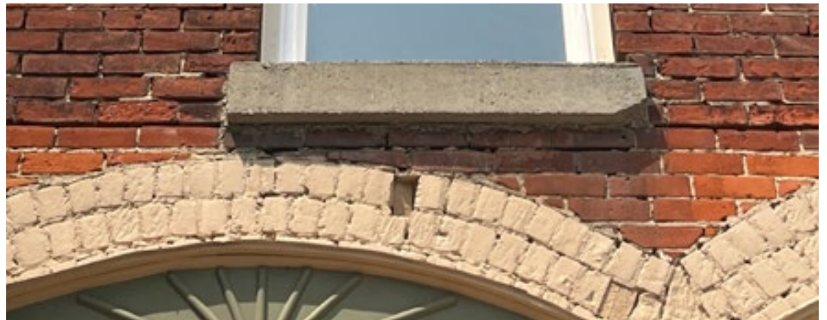
The mortar between the bricks on this building has degraded in areas. Proper maintenance of these historic materials is appropriate. Photo by KDG, 2023.
