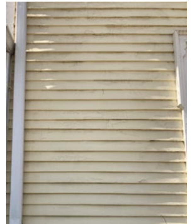
Remove damaged or peeling paint by hand scraping or hand sanding to the next sound layer and then repaint. Photo by KDG, 2023.
