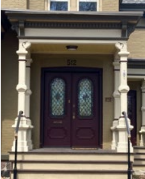
Historic features like these arch topped doors should be retained, maintained, and preserved. Photo by KDG, 2023.
