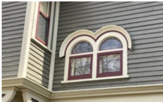
Regularly inspecting and repainting historic wood windows will ensure their longevity. Photo by KDG, 2023.
