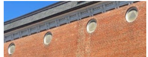
The protective glazing that was installed on these round leaded glass windows has yellowed over time and may have caused further damage to the historic windows. To avoid the pitfalls of inappropriate repairs, it is appropriate that routine maintenance and preservation of damaged features take place. Photo by KDG, 2023.
