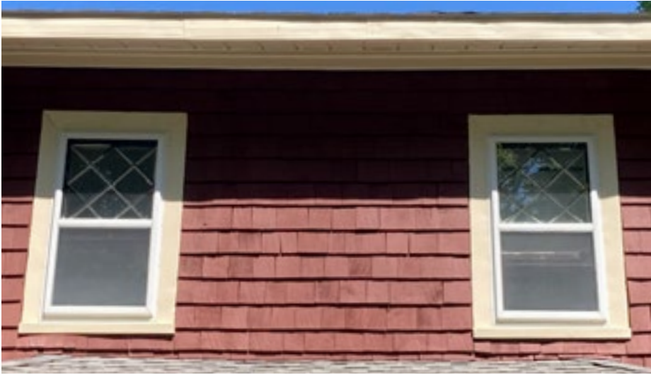
Routinely inspect and repair and repaint wood wall materials to ensure it stays weathertight. Photo by KDG, 2023.
