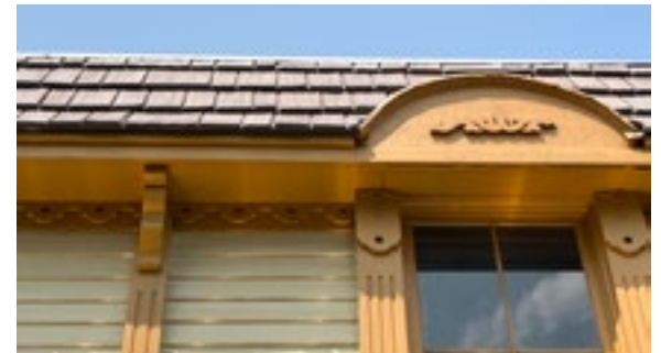
For commercial roofs historically covered in wood shingles, faux wood shingles that match the historic in terms of shingle dimensions, color, and texture, may be considered. Photo by KDG, 2023.
