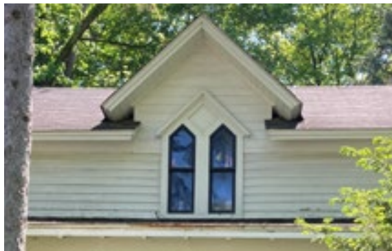
These pointed arch windows provide visual interest and historic character to an otherwise simply built home. Photo by KDG, 2023.
