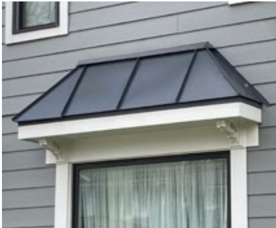
It is not appropriate to install metal seam roofing on a building that did not have it historically. Photo by KDG, 2023.
