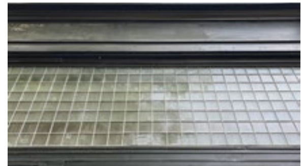
The historic leaded glass transoms above the large display windows on this storefront have been adequately maintained and preserved. Photo by KDG, 2023.
