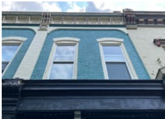
Details of an Italianate style commercial building along Main Street. Photo by KDG, 2023.
