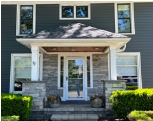
Removing or covering historic porch materials with new cladding is not appropriate. Photo by KDG, 2023.
