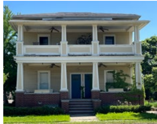
Inspecting, retaining and repairing historic porches and porch features is appropriate. Photo by KDG, 2023.
