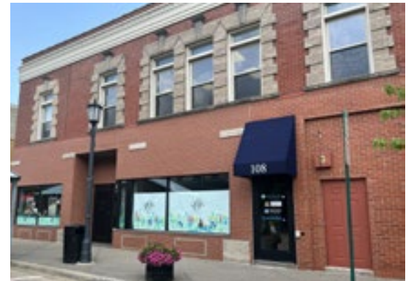
The appearance and pattern of the brick veneer on the first floor of the commercial building is distinguished from the historic brick on the second floor, indicating an alteration to the building. Photo by KDG, 2023.
