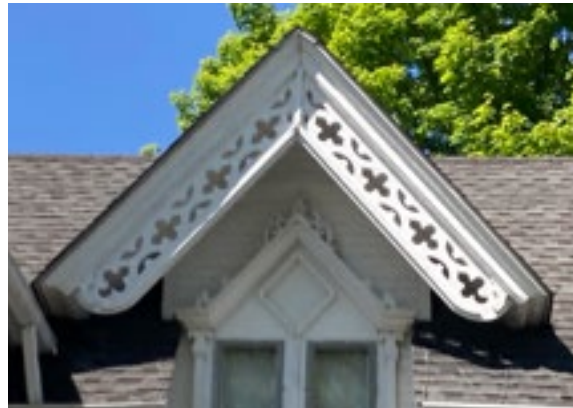
Decorative barge boards contribute to the historic character of the house and should be preserved. Photo by KDG, 2023.
