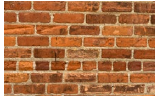
Maintaining and preserving masonry materials is appropriate and includes ensuring both the masonry units and mortar are adequately maintained, as shown above. Photo by KDG, 2023.
