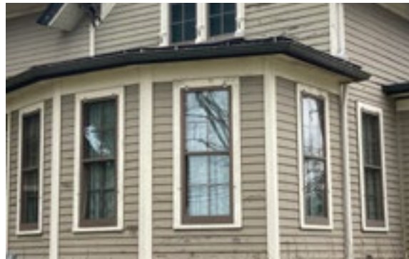
Installing storm windows that match the sash meeting rail of the window is appropriate. Photo by KDG, 2023.
