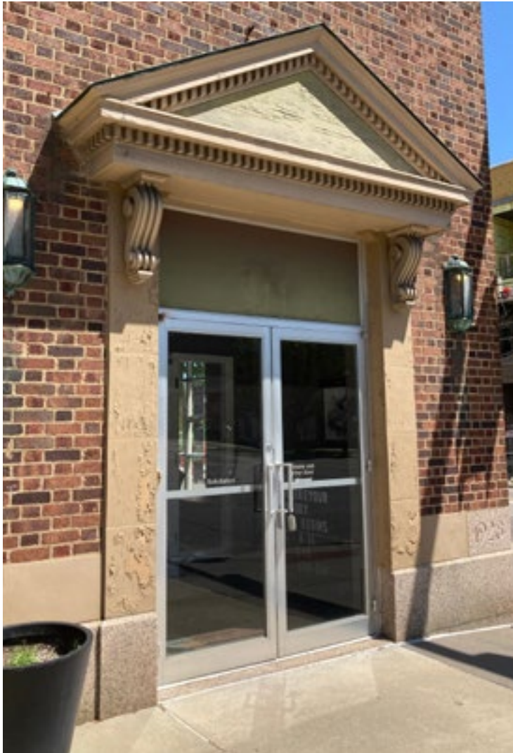
The aluminum exterior door system depicted above is incompatible with the historic character of the commercial building and is therefore not appropriate. Photo by KDG, 2023.
