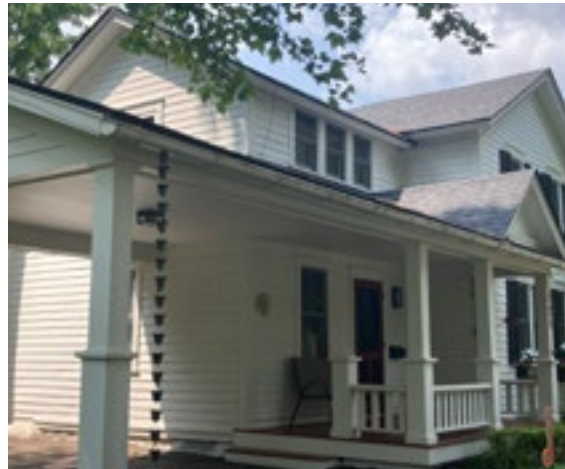
Gutters should be aligned with architectural features like the one seen here. Photo by KDG, 2023.
