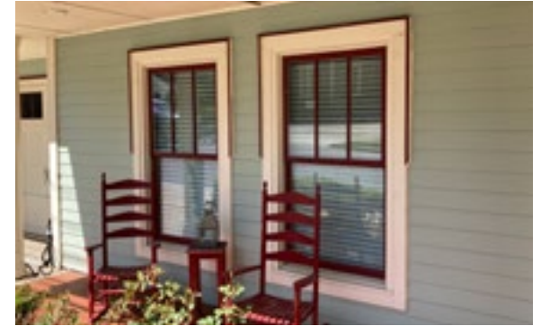
These historic three-over-one Craftsman style windows should be retained, preserved, and repaired. Photo by KDG, 2023.
