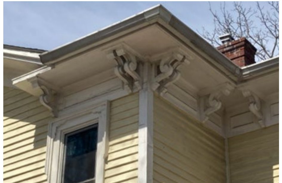
Periodically inspecting gutters and roofing elements ensures that issues are identified and corrected before they cause damage to the building. Photo by KDG, 2023.
