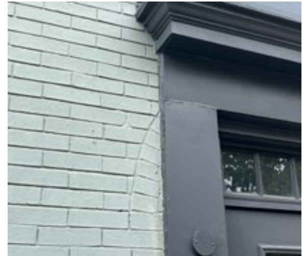
Arched brickwork indicates that at some point, an arched opening was altered to accommodate a rectangular opening surrounded by wood trim. Investigation into the building's history would help determine whether the alteration has acquired significance. Photo by KDG, 2023.
