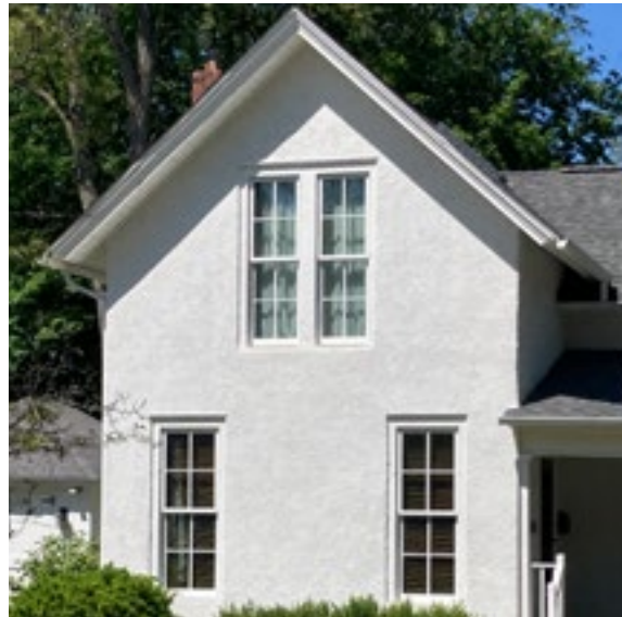
Determining the type of stucco is key to maintaining and repairing historic stucco cladding. Photo by KDG, 2023.
