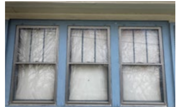
Although storm windows painted to match the window frame are preferred aluminum storms are acceptable. Photo by KDG, 2023.
