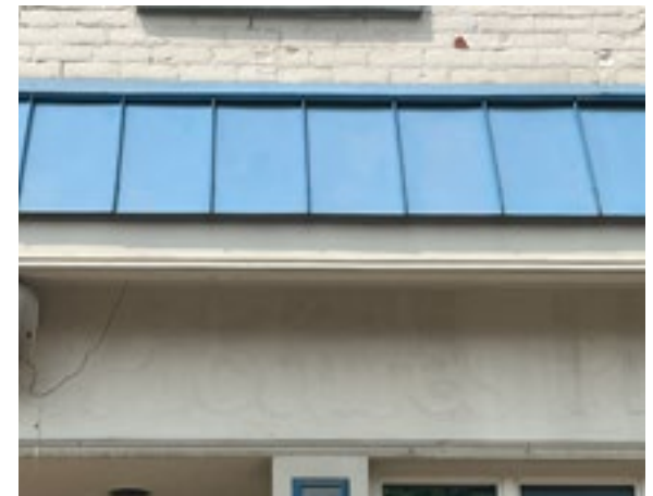
The pent roof above the storefront has been clad in metal roofing. Use of metal materials in this way is not appropriate. Photo by KDG, 2023.
