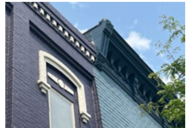
Architectural ornament, such as the window hoods, cornices, brackets, and cornice, is often highly decorative and part of the character defining features of a building, making the preservation of ornament important. Photo by KDG, 2023.
