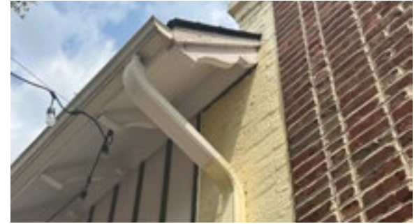
When gutters must be routed on the façade of a commercial building, it is appropriate for the gutters to follow architectural elements and be painted to match adjacent materials. Photo by KDG, 2023.
