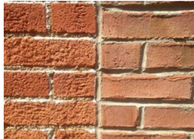
Abrasive cleaning methods like sandblasting permanently damages brick by removing the hard outer layer of the brick. This brick is now compromised and will allow water to leech into the building. Image courtesy of Jared Hyams and the Craftsman Blog (FaceBook).
