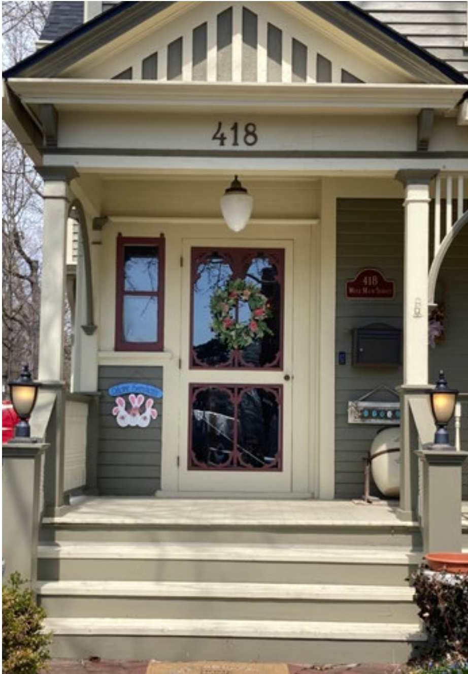
Proper maintenance of features and their materials prolongs their life. Photo by KDG, 2023.
