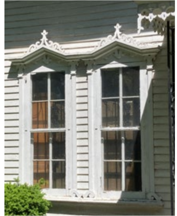
Window hoods and trim should be periodically inspected and repaired. Photo by KDG, 2023.
